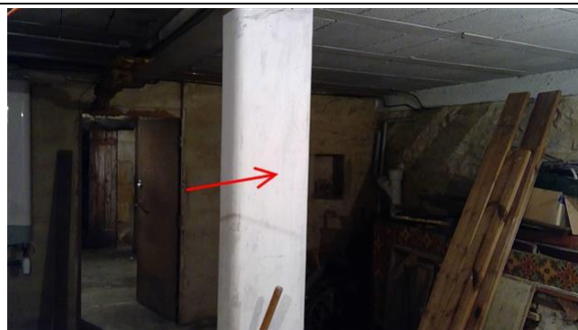
002 : amiante ciment Cave Cave (niv:-1)
