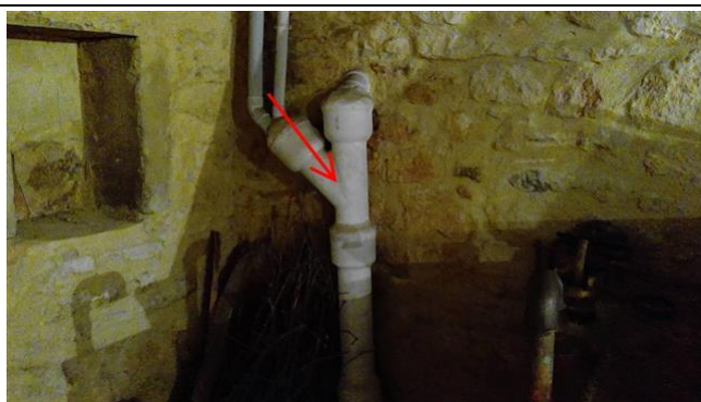
003 : amiante ciment Cave Cave (niv:-1)
